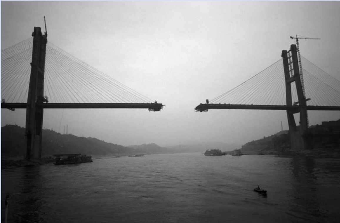
Suspension bridge under construction, 2002. A new suspension bridge is being constructed over the Yangtze River; the two sides of the bridge are coming together in the middle. (Photo from Justin Guariglia/Corbis.)
