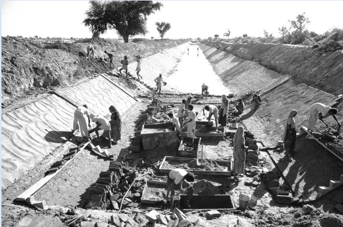
Building a main brick canal in India. Photo by Curt Carnemark, courtesy of World Bank Photo Library.
