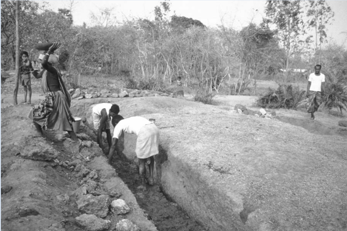
Workers digging irrigation ditch in India. Photo by Curt Carnemark, courtesy of World Bank Photo Library.
