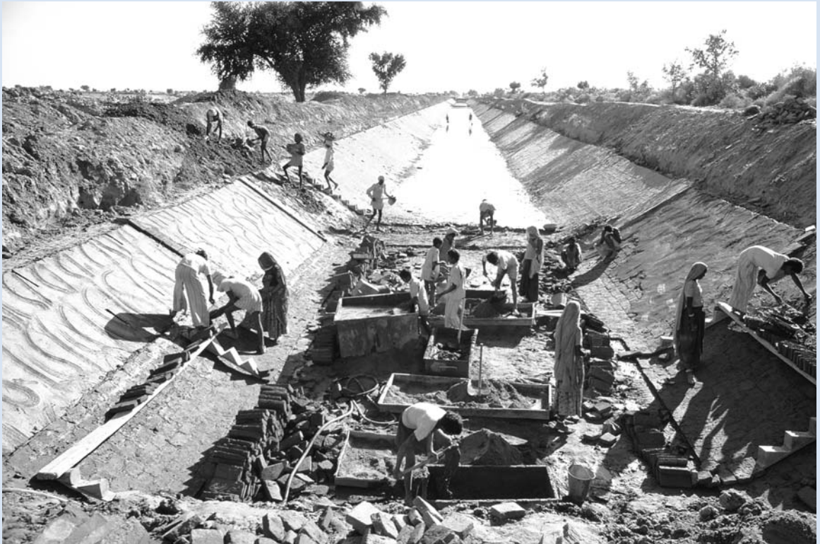
Building a brick main canal in India. Photo by Curt Carnemark, courtesy of World Bank Photo Library.
